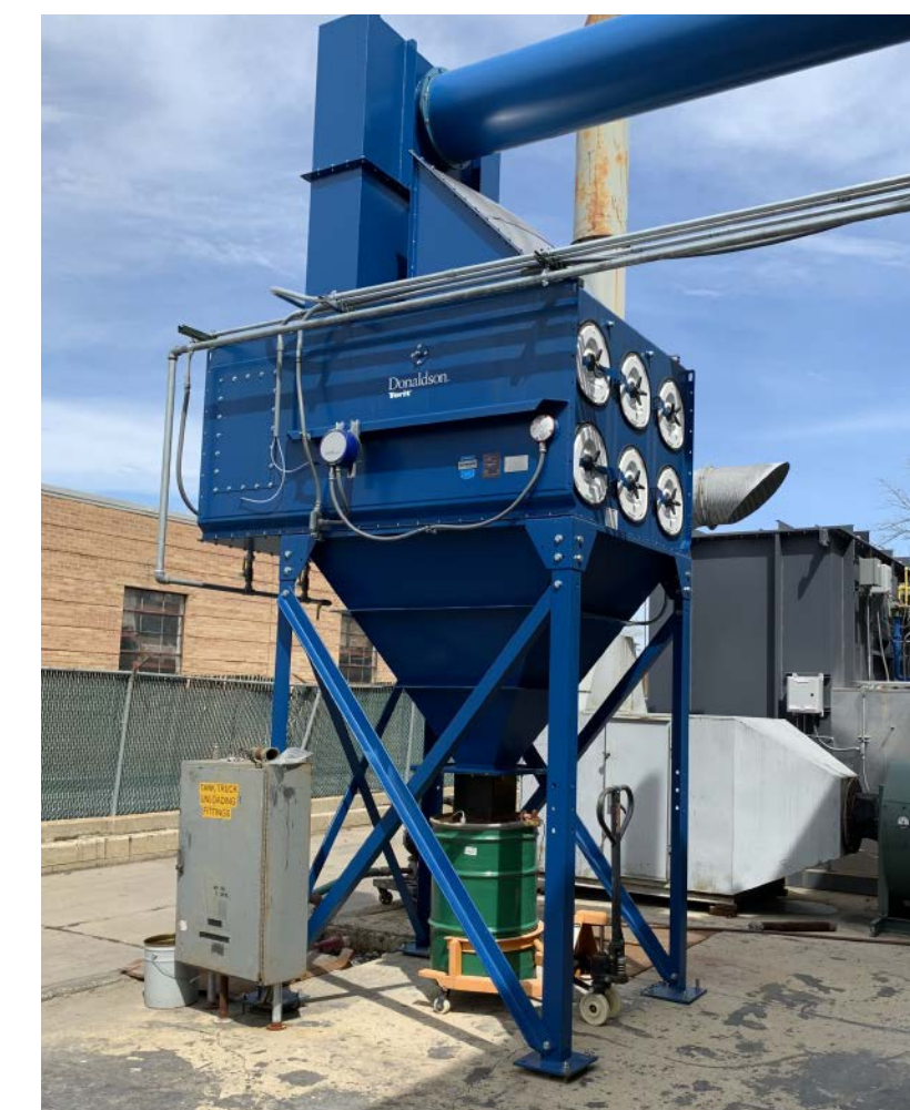
Dust collector, Chicago, Illinois.
