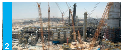
2 Sadara Chemical plant, Saudi Arabia. Estimated cost: USD 20 billion. Beckers product: 120 micron Beckry®Duro system.
