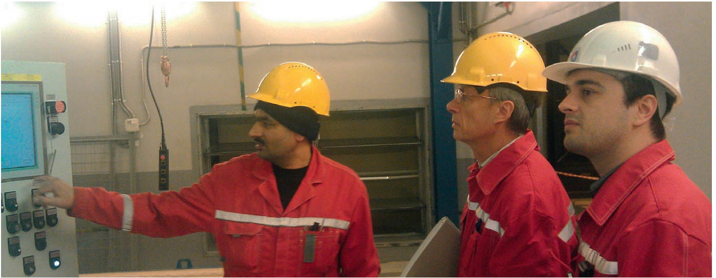
Start-up of Severstal's second line. Lage Holmberg and Yury Titovets from Beckers, with a Severstal supervisor.
